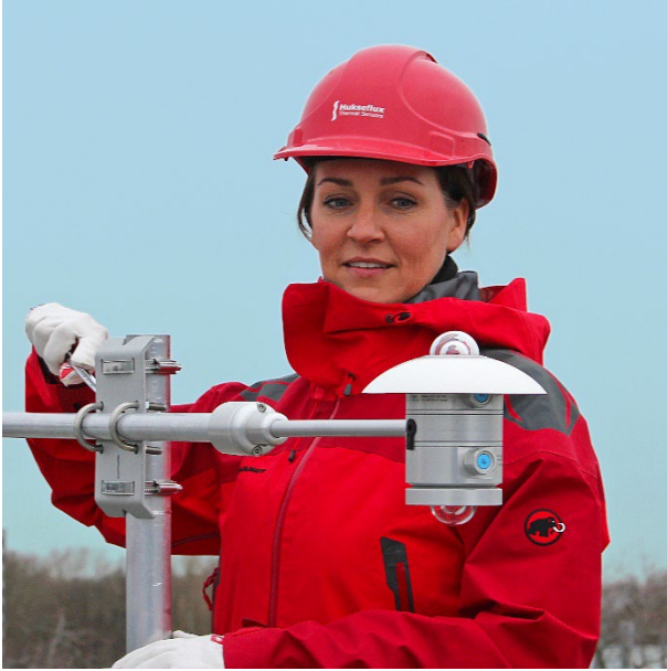
Figure 8 Installation of AMF02 albedometer mounting kit and two SR20 pyranometers, mounted with ALF01 levelling fixture on a crossarm with crossarm bracket CMF01.
